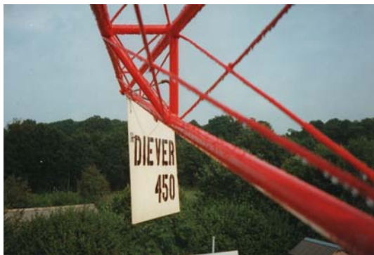
Fig. 6.6: vane hinge: 1" gaspipe, wooden bearings, vane locking device (photo 1994)
